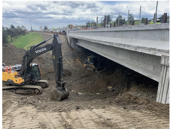
(Pictured Above: WB I-70 structure complete, crews beginning to grade shoulder and dig out underneath bridge.)
